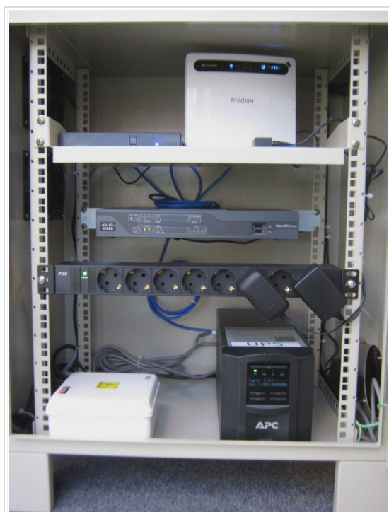
Fig. 2 - Interior de rack AD Rural
