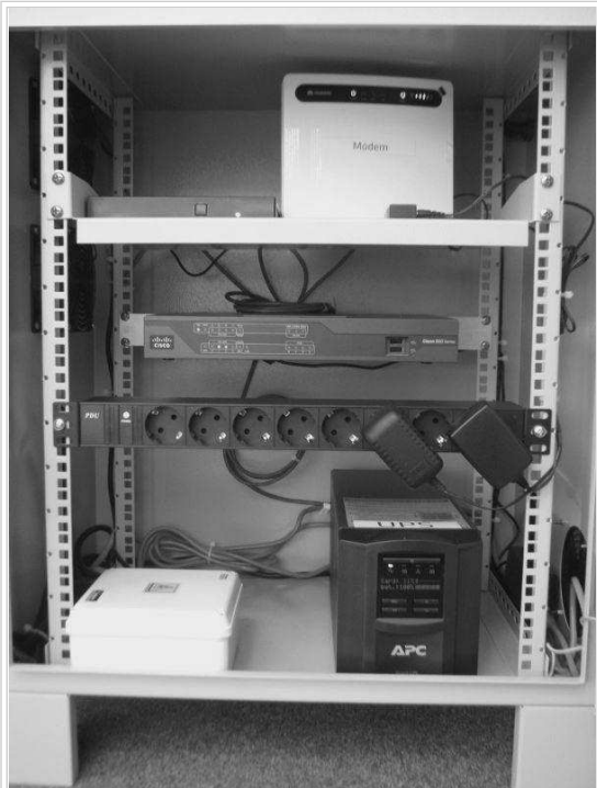
Fig. 2 - Interior de rack AD Rural
